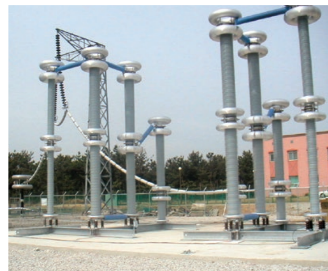
Fig. 4 Double-pole 600 kV outdoor HVDC test system type FGP 200/600
