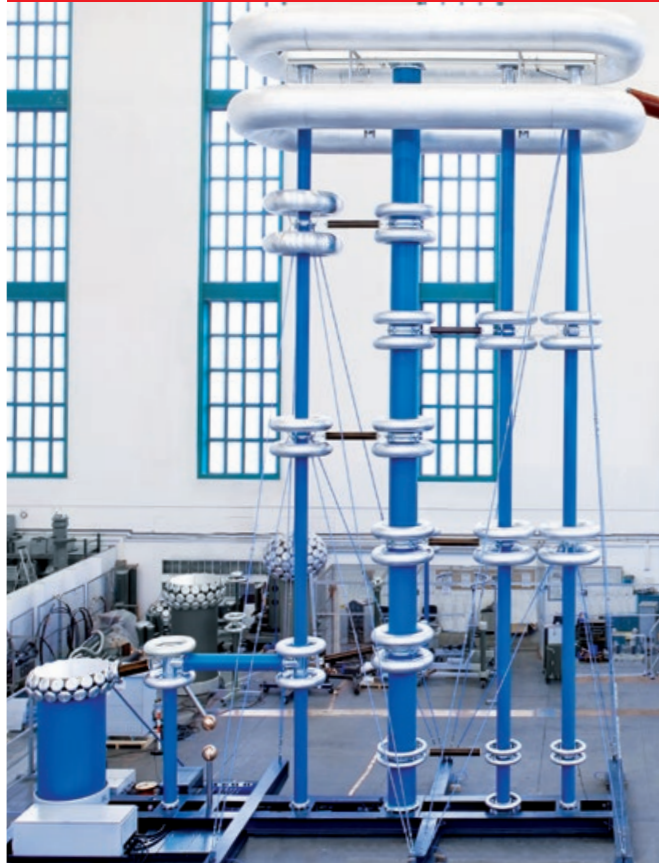
Fig. 1 HVDC test system type GP 50/2000
