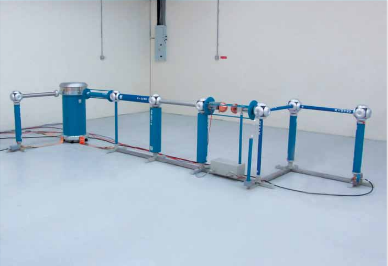
Fig. 1 Combined AC, DC, and impulse test system, type WGSBS 5.8/100-135-135, 100 kV AC, 135 kV DC, 135 kV impulse voltage
