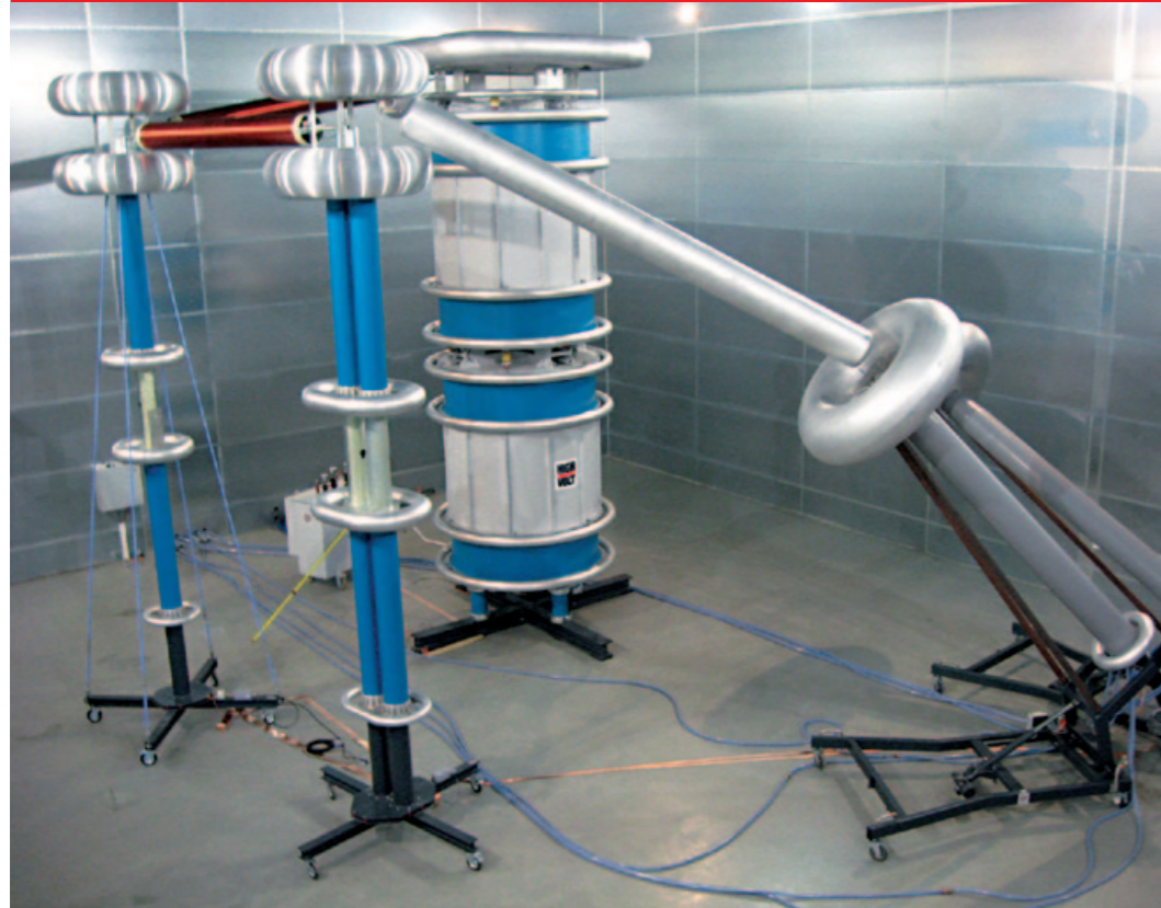
Fig. 1 Test field for 500kV cables with routine WRM test system with 800 kV and 28,000 kVA
