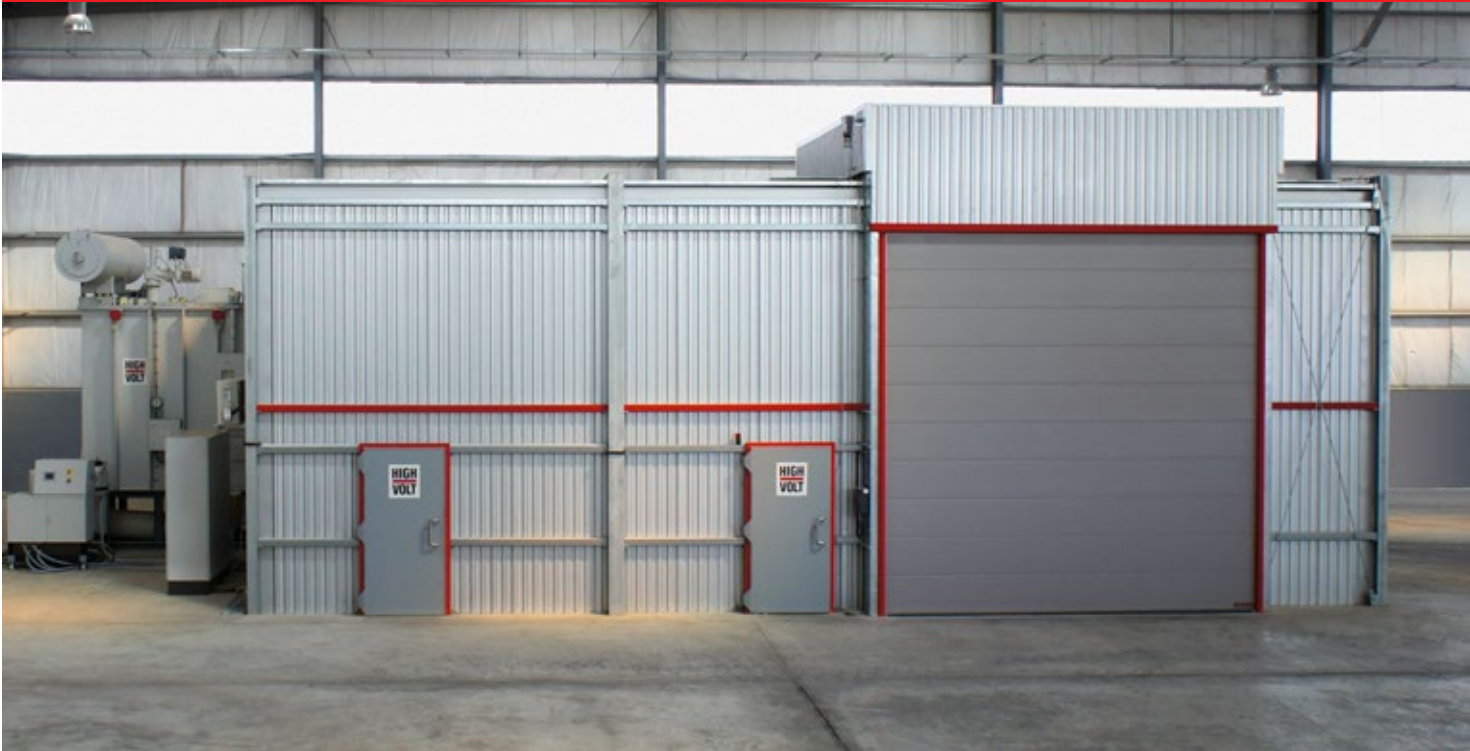
Fig. 1 Shielded room SSC 15x9x5.6 with integrated AC resonant test system WRU 10000/350-200-100 for routine testing of high-voltage cables
