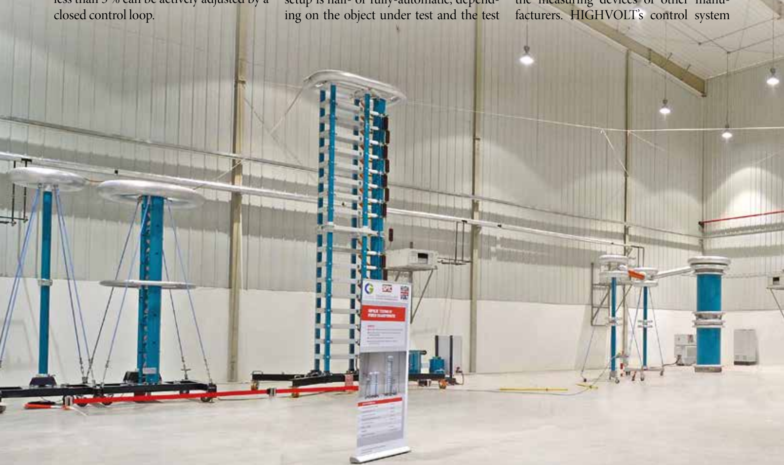
Transformer test bay with impulse voltage test system (left); AC test system with variable frequency (centre); and transformer loss measuring system LIMOS and HV-filter (right)
