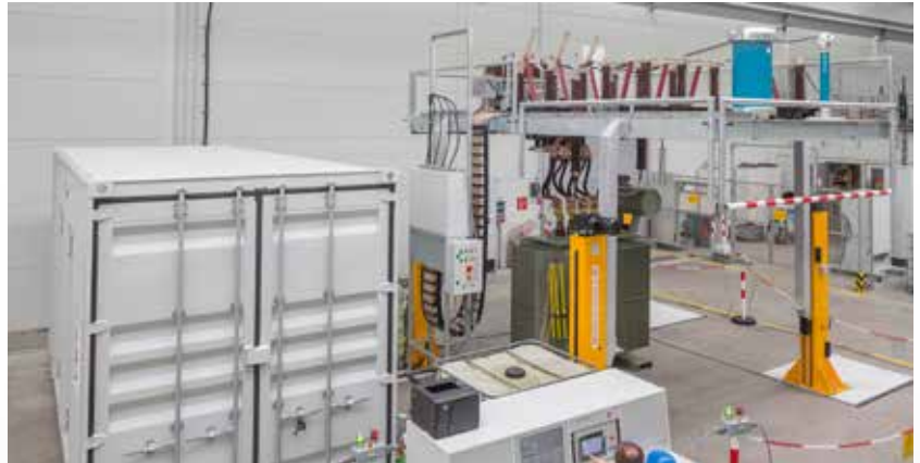
Container raised static frequency converter with a movable platform for easy connection and testing. One particular advantage of the test system is its automatic operating mode, in which all of the internal settings are pre-selected on the basis of the corresponding test data set. The control system is characterized by a user-friendly intuitive handling.
